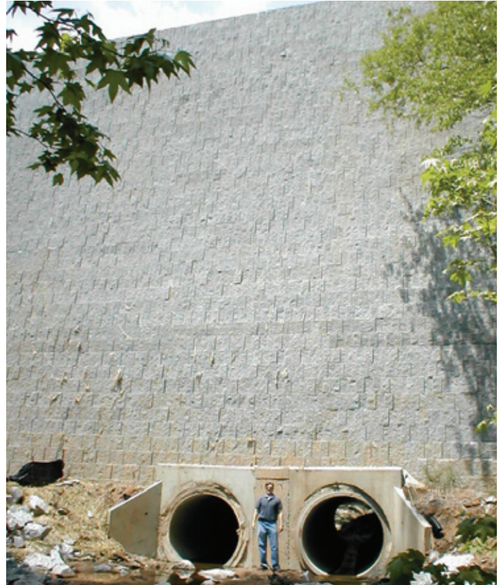
To provide drainage, the land bridge structures have two six-foot-diameter culverts through the 61-foot-high walls.
