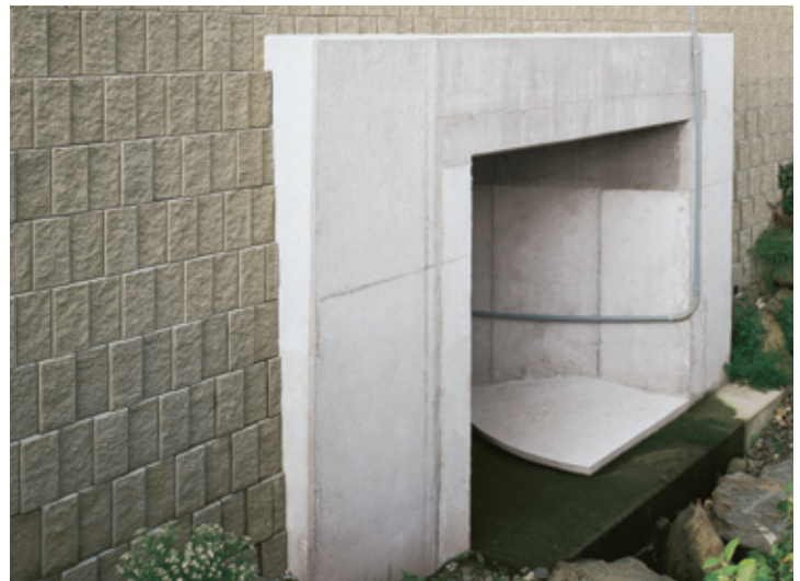
The wall design was changed so that there was safe access to the water utilities after the wall was constructed. That meant project work could proceed without utility delays.
