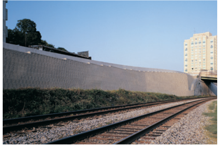
The unique direct-anchorage option of the Landmark retaining wall system made it possible to relieve pressure on an existing MSE and stabilize the structure.
