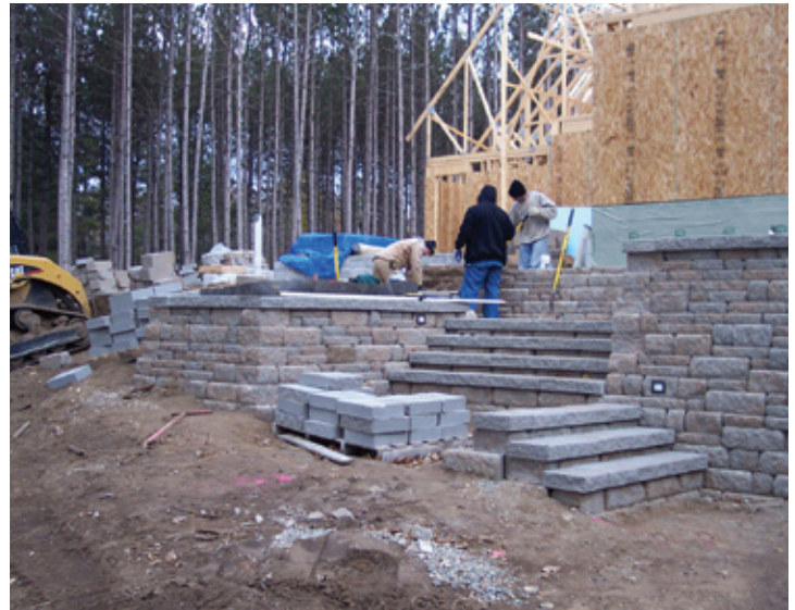
The contractors designed and built the home's landscape before the house was completed.
