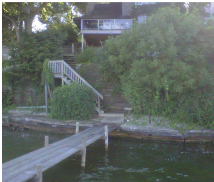
A rotting timber wall and slippery steps made access to the lake on the steep slope dangerous.
