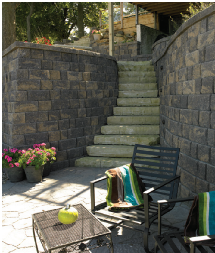
Terraced retaining walls transform a steep, dangerous slope on a small lot into useful, safe and beautiful landscape.
