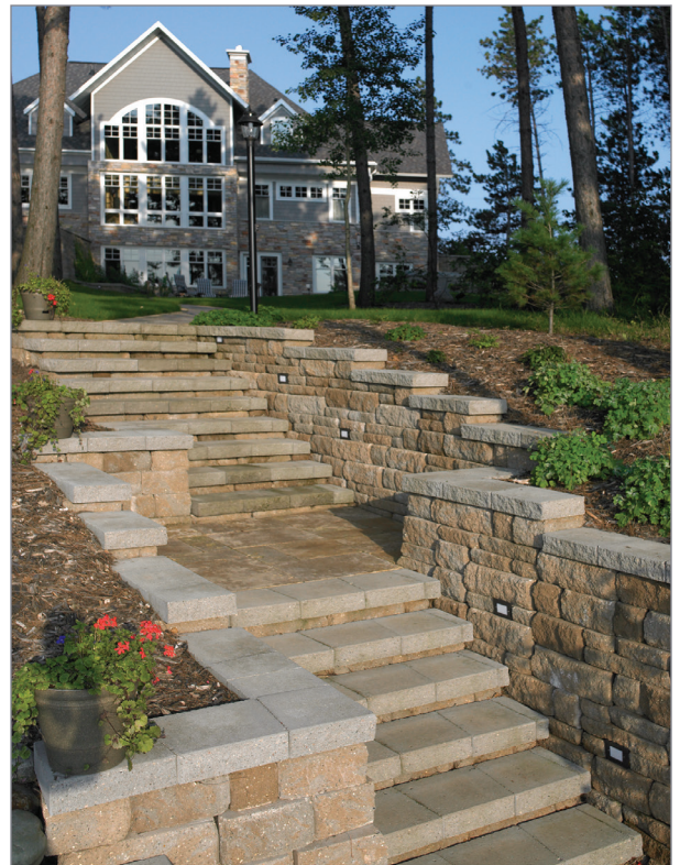
The hardscaping continues with paved steps and a walkway and a Highland Stone® 6"/3" retaining wall leading down to the lakeshore.
