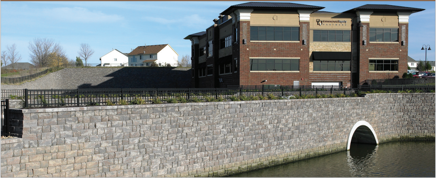
The Diamond Pro Stone Cut® retaining wall system features a custom-design drainage pipe in the detention pond.
