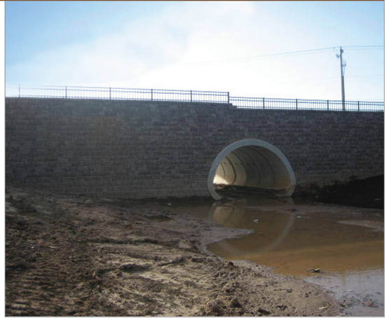
The contractors needed to build the detention pond quickly, before it filled with storm water.
