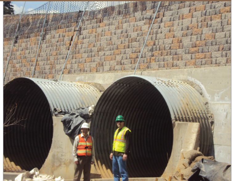
The challenging installation of this 65,000-square foot retaining wall occurred at the bottom of a slope and above a creek.
