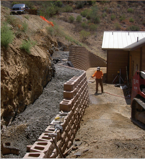
Construction is under way using the Anchorplex™ retaining wall system which significantly reduces the excavation commonly associated with segmental wall systems.
